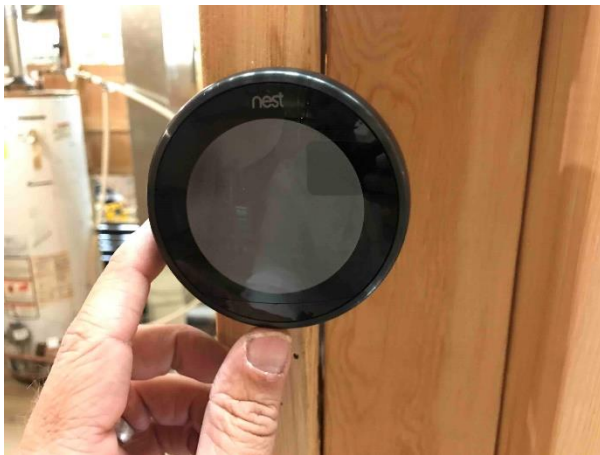
Image of a high-efficiency thermostat at the InterNACHI® House of Horrors® in Colorado.
